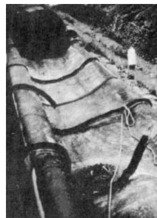
Pipe damage in power station Okigawa
